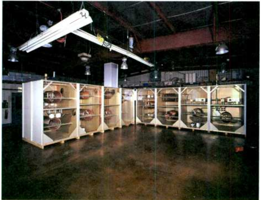
200kW x 200kW (400 kW total power) diplexer
