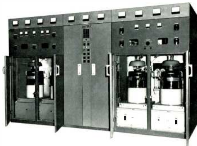
Three main transmitter cubicles house (from left to right) the modulator, RF driver, and power amplifier.
