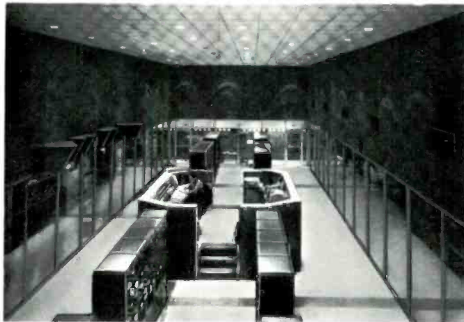
VOICE OF AMERICA—Six Gates 50,000 watt Model HF-50C transmitters are in use at the Greenville, N.C. transmitting station.
