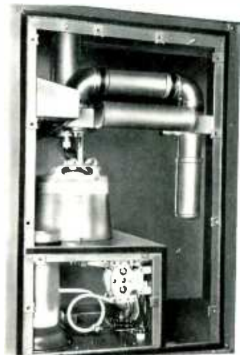
The Power Amplifier stage, which uses a 4CX15000A ceramic tube, has its driver amplifier located directly below for added efficiency of operation.
