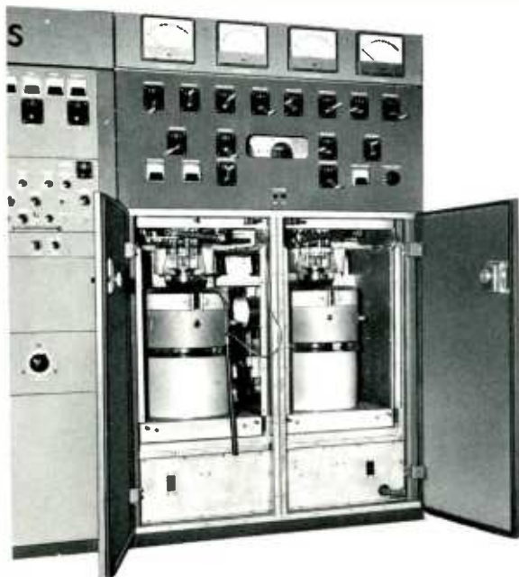
Front view PA cubicle with internal shields removed.
