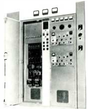
The exciter is located in the center cubicle and also includes the heart of the control system as shown above. There is sufficient space for optional dual exciters permitting operation on twenty crystal controlled channels where desired.
