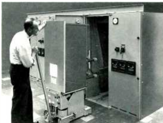
One of several 4160 volt primary power breakers with 150 megavolt ampere rating.
