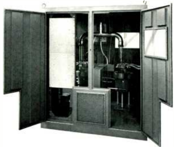
Modulator cabinet showing 4CV100,000C tubes and vapor phase cooling system.
