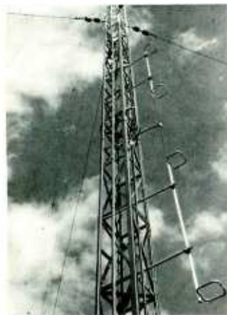
RA-4 Base Station Antenna.
