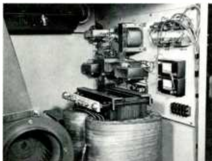
Power supply assembly (bias, screen and plate) can be reached quickly. Husky transformers invite 24-hour schedules.
