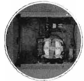
Below: A single solenoid relay in the Conelrad RF cubicle is push button operated to change from the main RF section to Conelrad.
