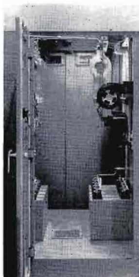
Rear view of HV rectifier cubicle. Long life, trouble-free vacuum tubes are in "walk in to service" surroundings.
