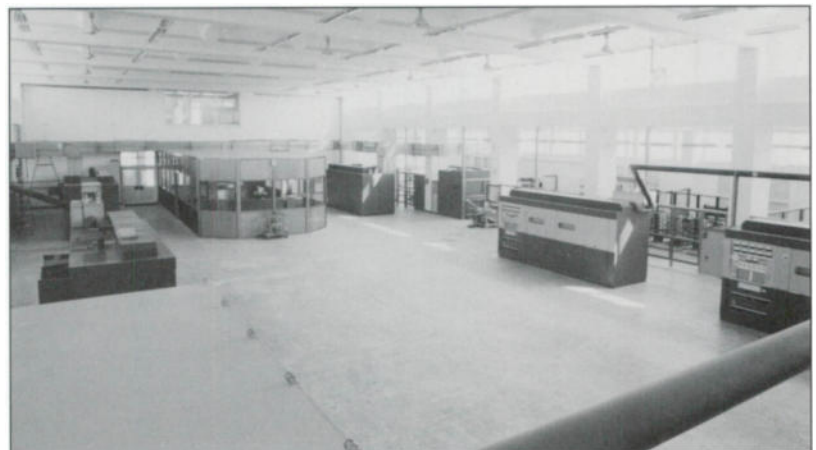
High power broadcast facility in Taiwan housing 300 kW MW transmitters and 100 kW SW transmitters.
