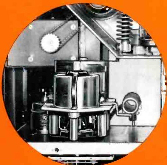
21M POWER AMPLIFIER RF CHASSIS
