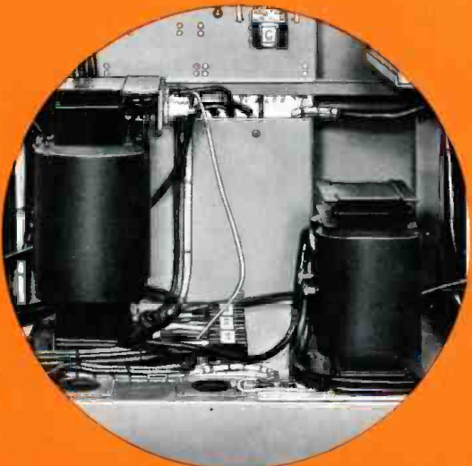
POWER SUPPLY CABINET MODULATION TRANSFORMER
