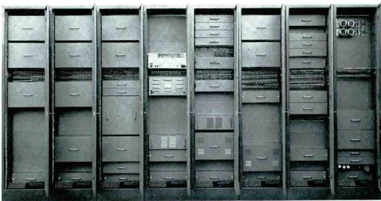
Rear view master control rack equipment — custom built for AM-FM operation
