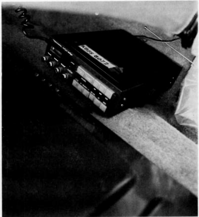
Another good spot is the storage area in back of the driver's seat. All the wire and coax runs will be short, but you may have to punch through the truck's body if your truck is made of single-wall construction.
