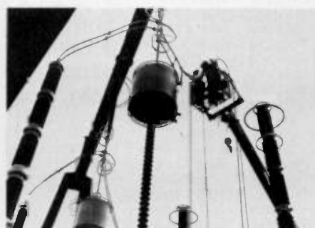
Electric power utilities, such as the one which brings you electricity, all maintain emergency crews to cope with accidents, blackouts, and the adverse affects of the weather. These crews operate 'round the clock with "electrifying" communications you can hear on your scanner!
