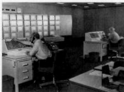
The nerve center of the entire Tennessee Valley Authority power system is the Load Control Center in Chattanooga; dozens of communications frequencies are in use here.
