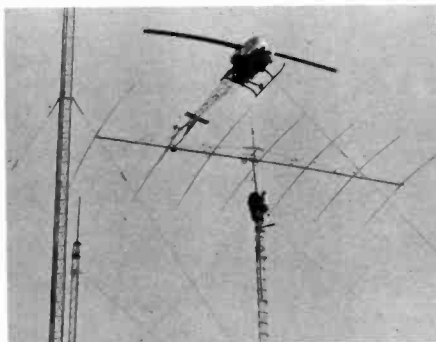
Amateur antennas come in all sizes. This one required a helicopter to raise it into place.
