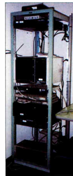
CNI's equipment rack in Cablevision's office
