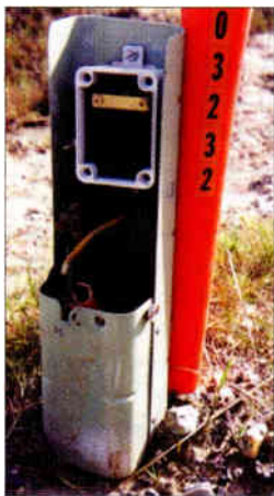
Figure 4: Above-grade access to cable armor.
