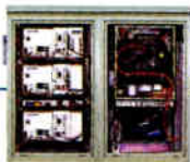
CPS-1 2.7kW w/ N+1 & Generator
