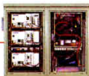
CPS-1 2.7kW w/ N+1 & Generator
