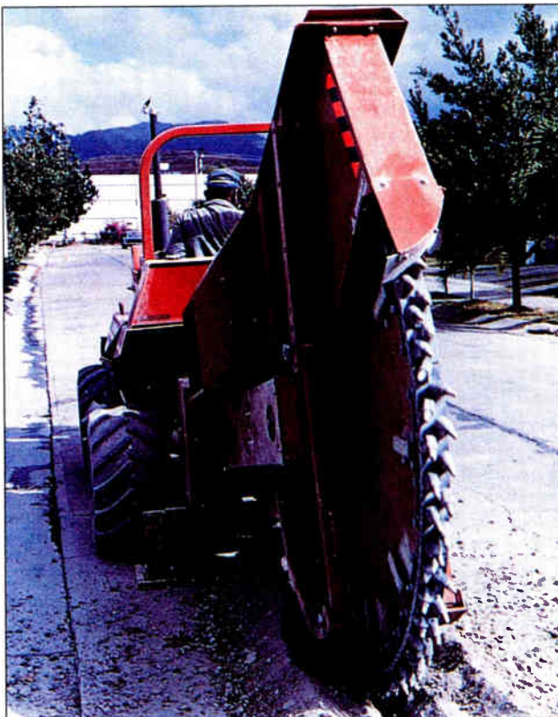
Placing underground cable in conduit allows CATV operators to avoid the costly trenching process when replacing cable or upgrading to fiber.
