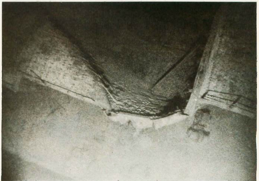
Photo 4: An area of major damage between the first and second smokestacks.
