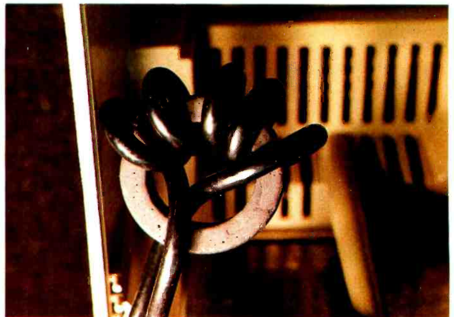
Photo 8: To reduce any high-frequency harmonics that might radiate from the video-monitor cable, a toroidal ferrite core may be wrapped in the line.
