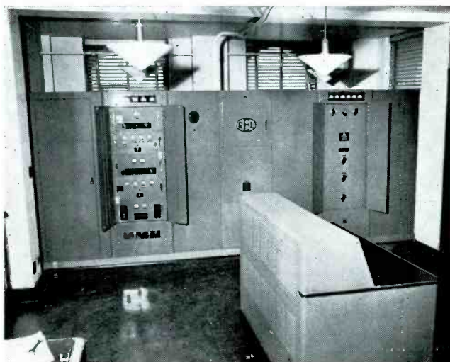
Modulator unit, intermediate power amplifier, driver, and power control console at WENA. The output of this unit delivers 3KW to the final amplifier.
