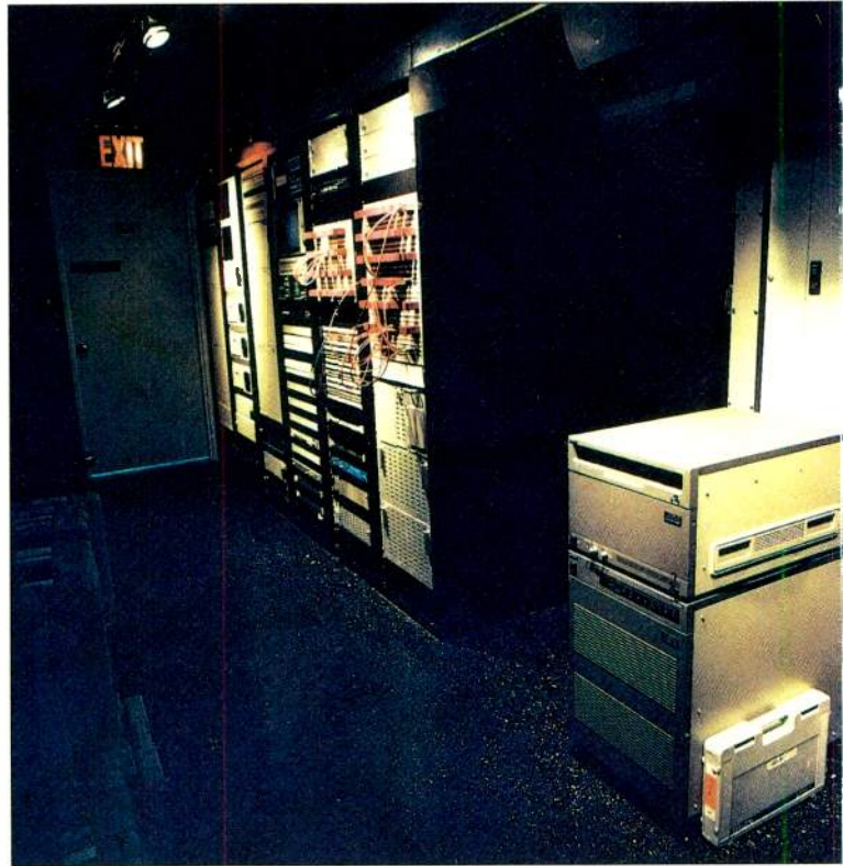
Completed and operational machine room at Image Mix.
