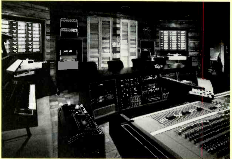
Studio A at Omega Studios' brand-new Rockville, MD, recording facility measures 50 by 40 feet, with an 18-foot ceiling—large enough to house orchestras and choirs, even at the same time. The control room, pictured here, features a 56-input, 48-output API console with FADEX. Other equipment includes Dolby and dbx noise reduction, Studer ATRs, Q-Lock synchronizer, Sony VTRs, and reverb and signal processing gear, as well as an array of traditional and electronic musical instruments. Omega plans conversion to digital audio in the near future for Studio A as well as its Studio B.
