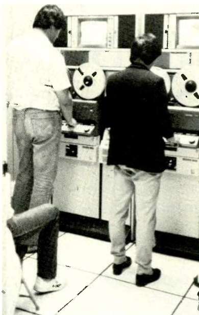
One of the 18 one-inch edit bays within the master control complex of the CIR. All are equipped with Ampex VPR-6 VTRs.
