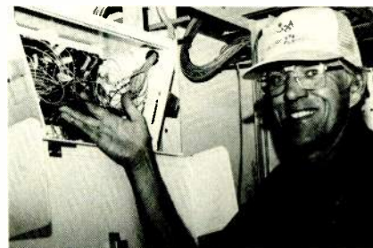
Lyle Bradt displays fiber optic cable in Pacific Bell's mobile telecommunications facility at the Los Angeles Coliseum.
