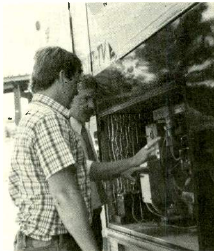
Supervisor of special engineering Marvin Mitchell, left, and engineer Jeff Nelson examine the generator in the Newstar truck. Newstar can also use shore power.
