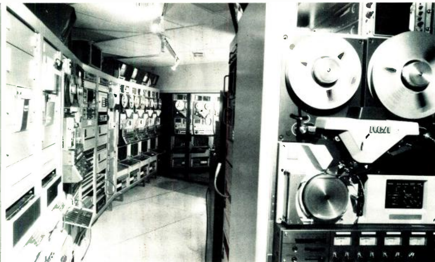
Central equipment room houses the RCA and Sony one-inch VTRs.
