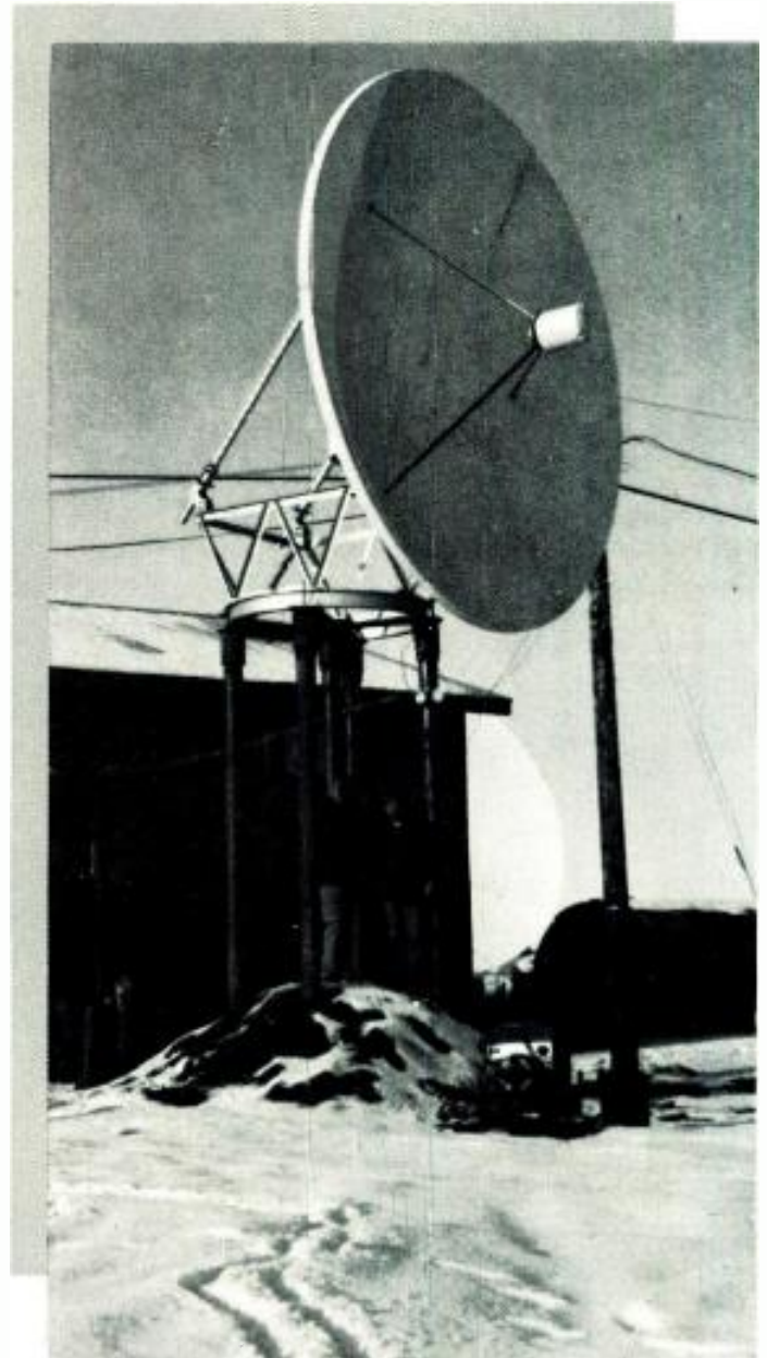
NPR dish at KOTZ in Kotzebue, AK has nearly zero elevation angle to point to satellite, far south.
