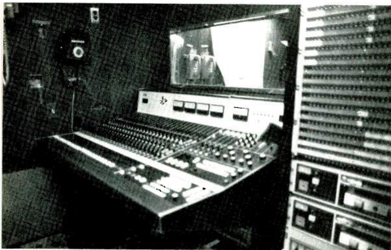
24 input Ward-Beck Systems audio console was installed during the basic construction of the trailer itself since it was too large for later installation.
