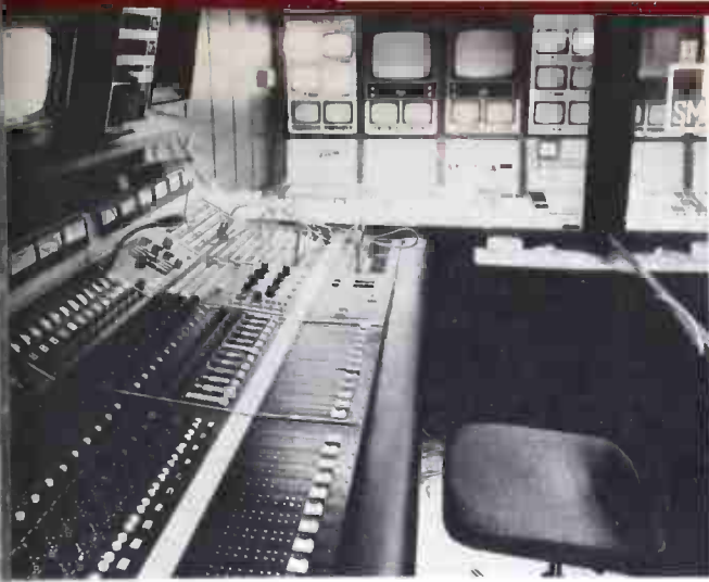
Audio control position for mobile studio, looking forward toward video monitors, etc.
