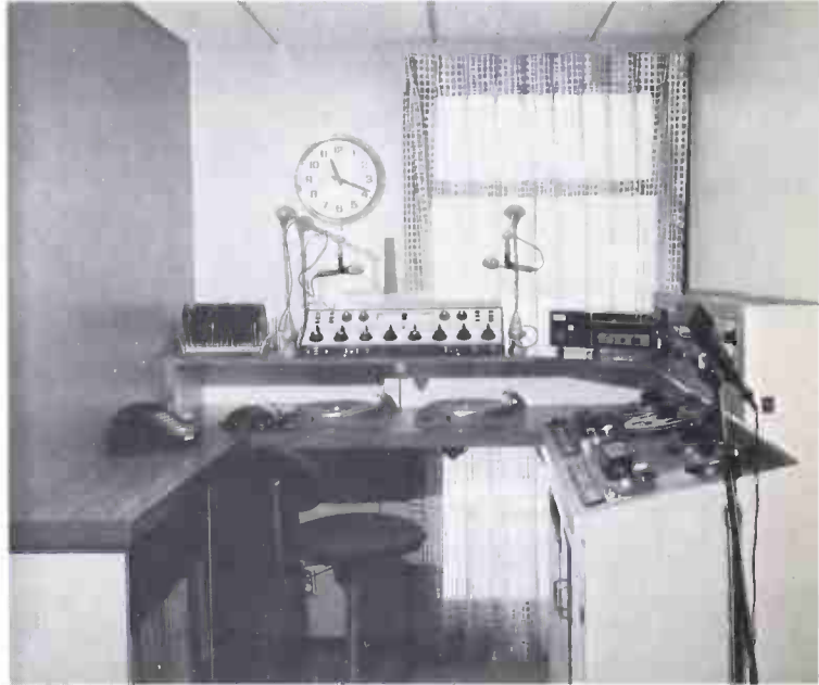
One of two identical stereo production rooms at KMWX-KFFM—which could be used as a control room.
