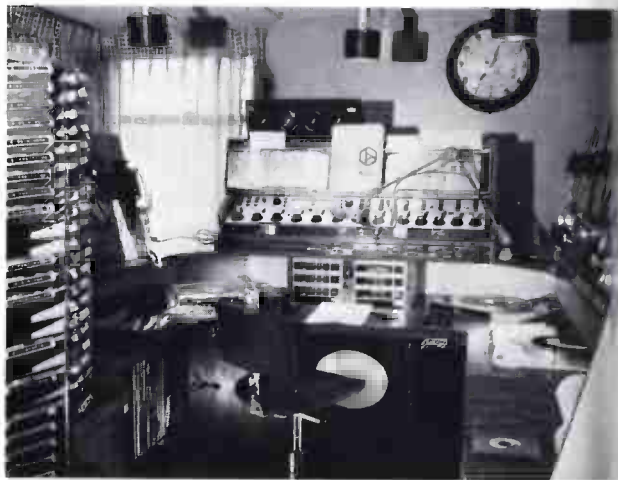
This is the Master Control Room. The five pots, 25-button extender panel on the Sparta console (right side) eliminates need for patch panel. The six ITC cart machines operate in sequence.
