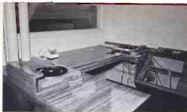
Production Studio A during the early construction stage, showing location of turntables. Ampex PR-10's go into right-hand sloped panel. Carts are in left-hand extension. Through the studio window you can see the master control room.
