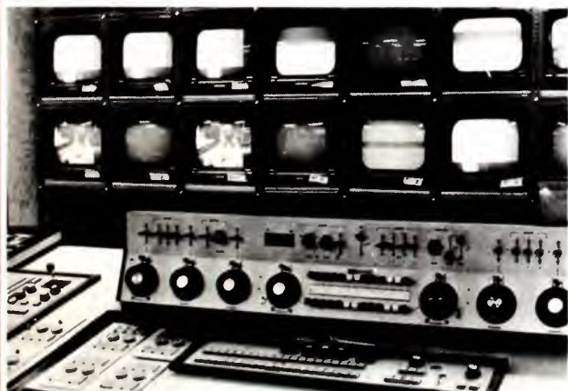
Master control room also serves as Studio A control. Remote switching panel (below Gates audio control) makes it possible to handle Studio A production and on-air signal. CCU, sync generator, DAs, etc., are directly behind switching console.
