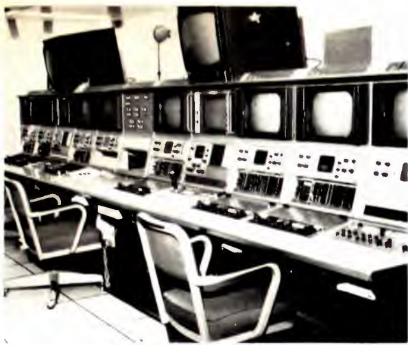
Camera control units and video processing section in master control.
