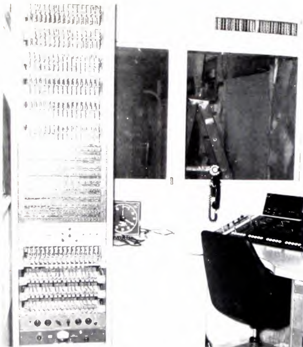
Rack at left holds most of electronics of audio system, including line and booster amplifiers, light-controlled fader units, equalization, etc. Console at right has remote-control faders, switching.
