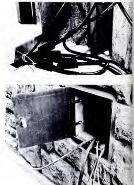
(Top) Cableraceways at all conceivable camera positions keep cable from being exposed to view. (Bottom) The mobile unit can be hooked up to the sound system in the cathedral from the outside, eliminating the laying of cables.
