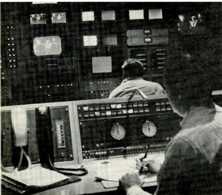
Master control uses IBM-card-controlled automation with manual override at any time. All program sources are available here for instant changes.
