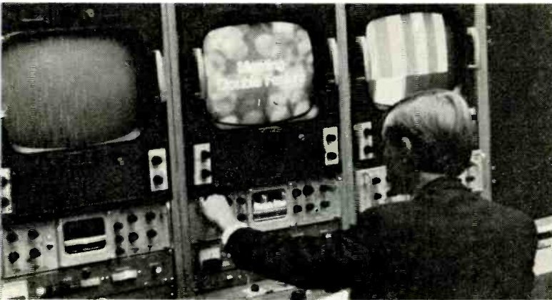
Terminal equipment room contains station's audio and video distribution facilities, sync generators and camera controls.
