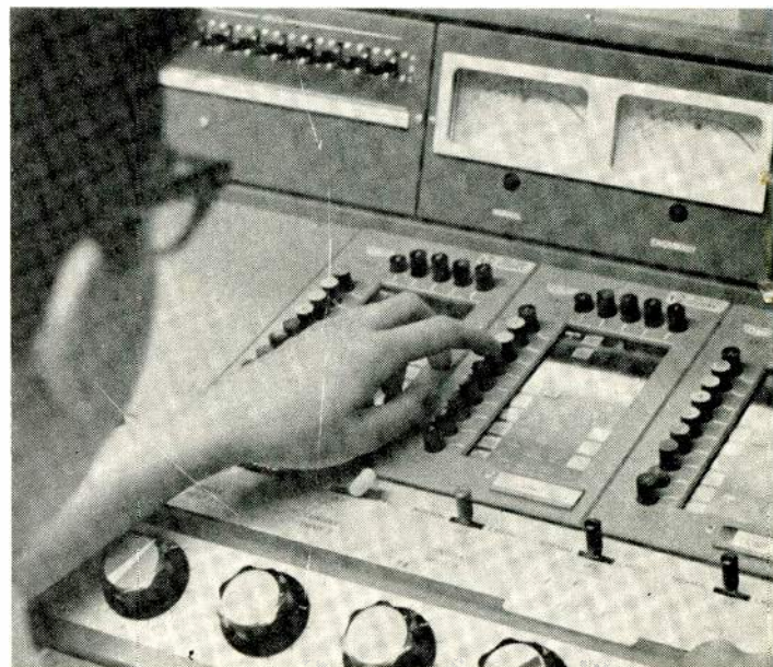
Crossbar switching shown close up above, has eliminated patch cords once and for all. Crossbars are duplicated throughout studios, even on newsdesk (right) for "patching" in phone calls.
