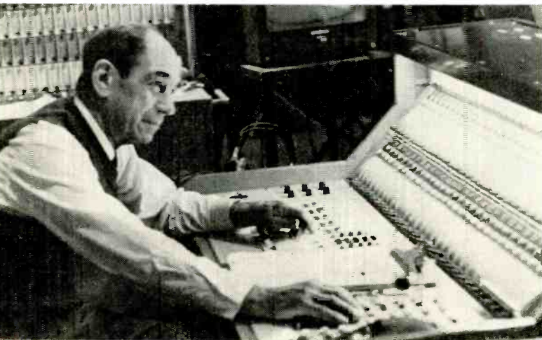
Solid-state studio lighting control board by ColorTran lets one lighting specialist handle Studio 5's 200-plus quartz lamps.
