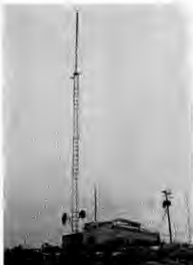
Radome-covered microwave dishes are mounted on the TV tower at both transmitter sites. Shown here is the KNDO-TV transmitter building at Ahtanum Ridge.
