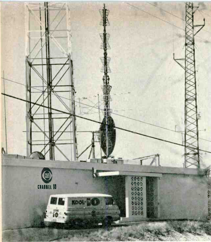
Mt. Suappoa KOOL-TV transmitter site. Microwave signal is transmitted via a 10' parabolic antenna (mounted on center tower) to Pinal Peak, a distance of 72 miles.
