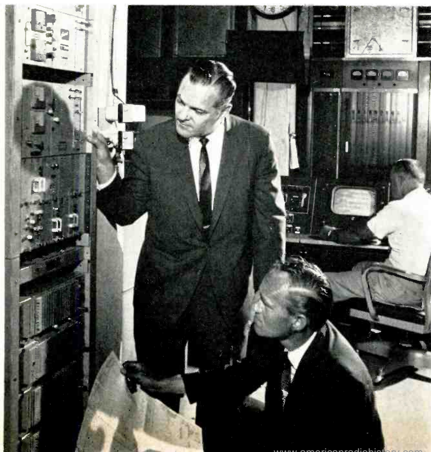
Authors Hillstrom (r) and Layton examine Lenkurt 76TV equipment at Mt. Bigelow KOLD-TV transmitter site.
