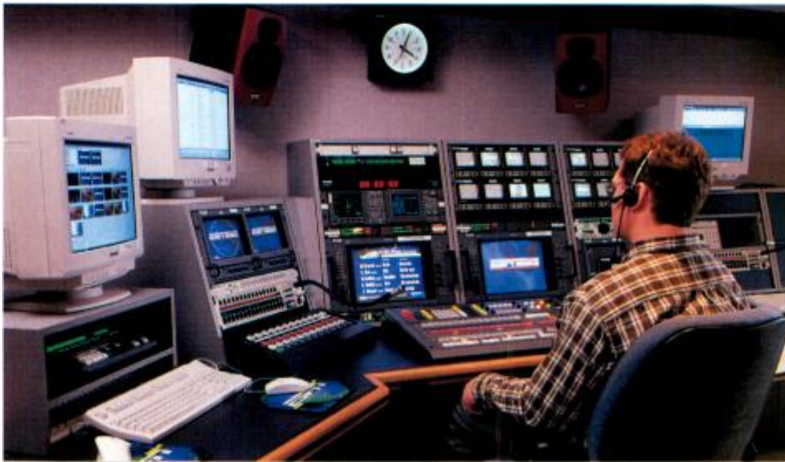
Audio Control Room 9 allows a single operator easy access to critical on-air devices and line-of-sight access to the director.
