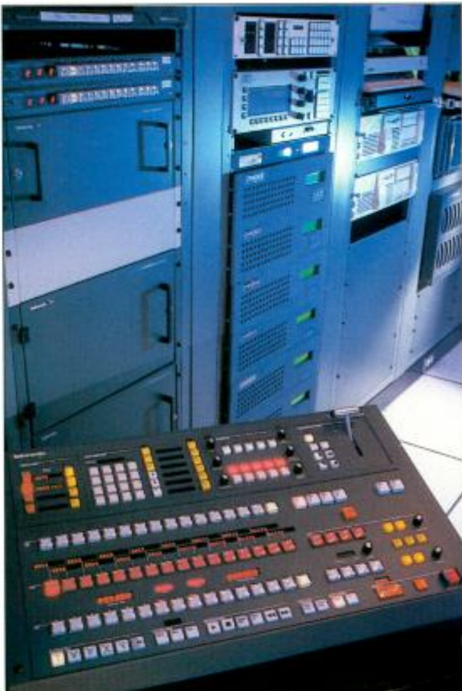
A pair of Grass Valley M-2100 master control systems and OmniBus automation provide the control needed to direct both HD and multichannel operations.
