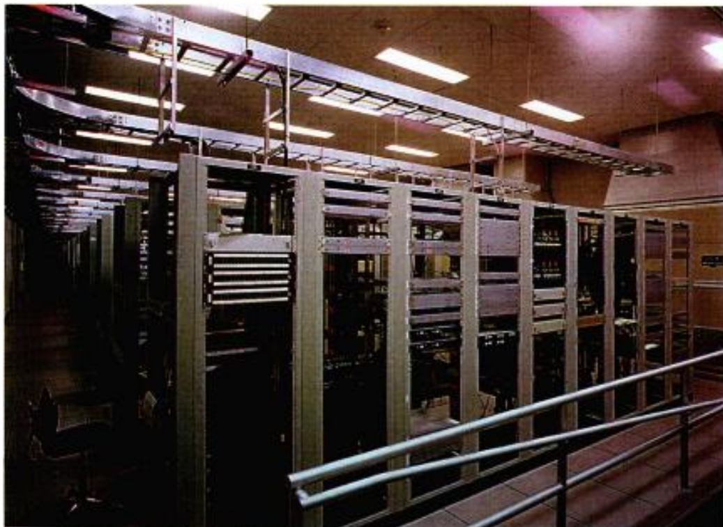
Rack and equipment rooms only get smaller. It's crucial to build them larger than initially needed if there's to be room to grow. WJXX-TV technical room begins with 12 rows of deep racks.
