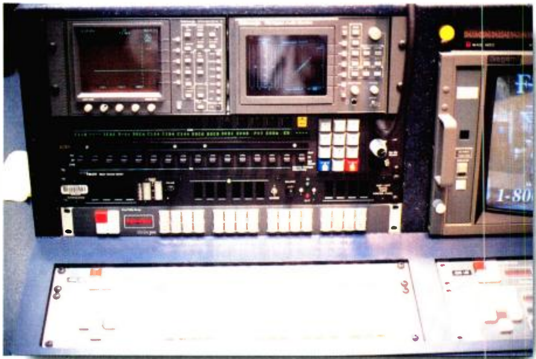
Maintenance of digital systems will be more centralized than ever. Test stations like the one shown here will concentrate sophisticated test equipment at one location where signals can be carefully analyzed.
