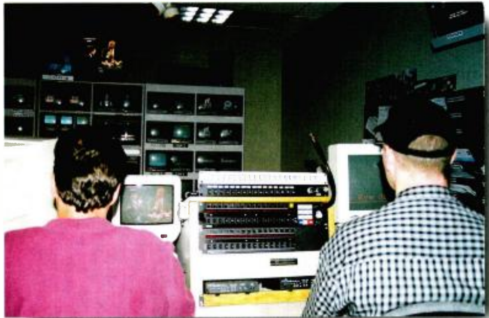
The "B" control producer's station, shown here, provides full communication to both local and remote locations (some 30 miles away) through the new Telex Adam intercom.
