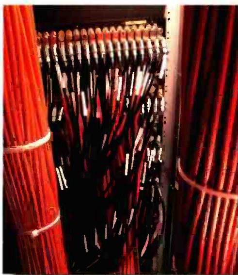
The new digital station features a comprehensive cable management system with more than 3,000 cables clearly identified and mapped.
