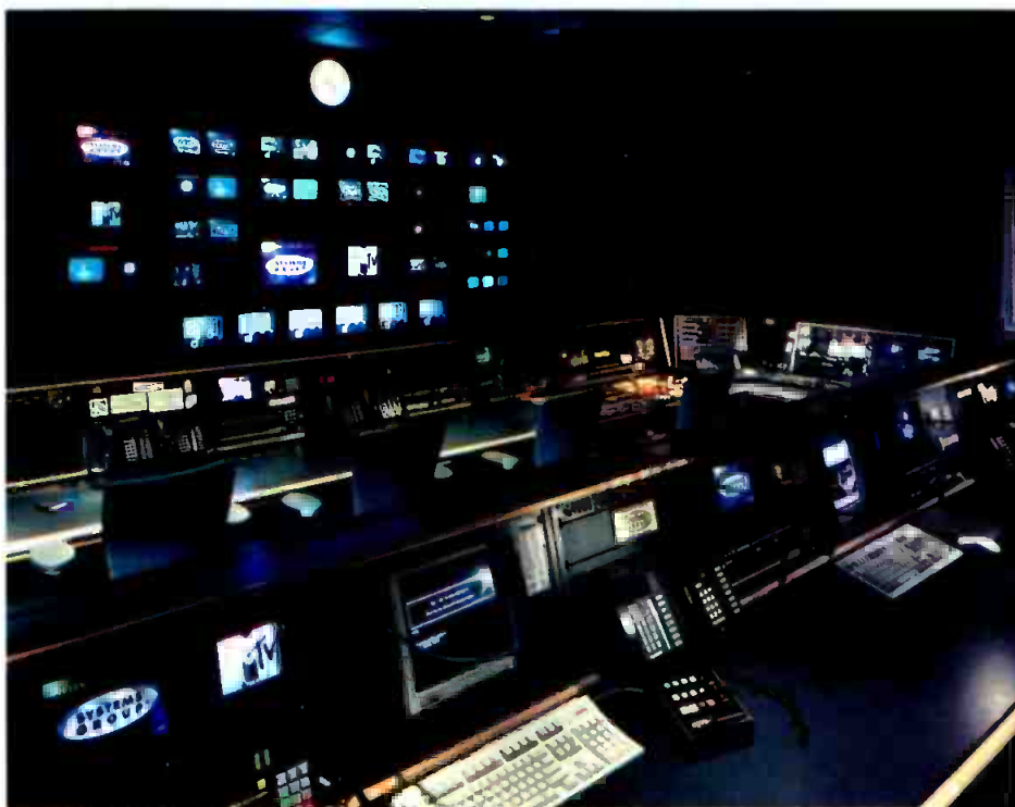
The control room is based on a Grass Valley Group 4000 digital switcher with access to five studio cameras and three remote cameras. The work area provides space for a director, technical director and three producers.
