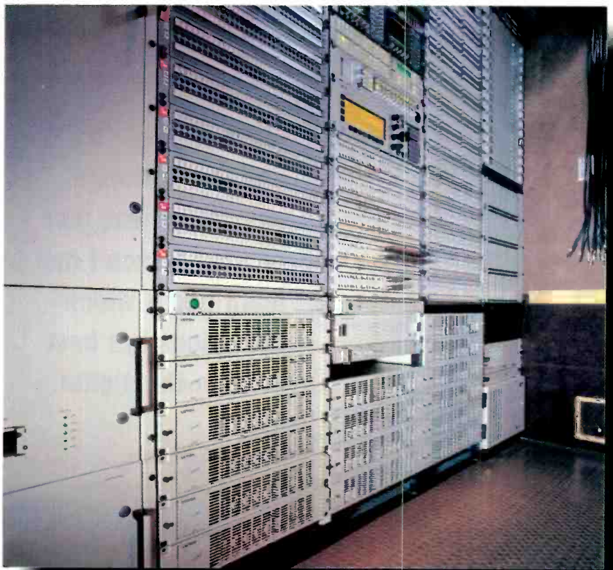
Doc Holiday's control center, featuring many racks of Leitch DigiBus and Digital Glue.
