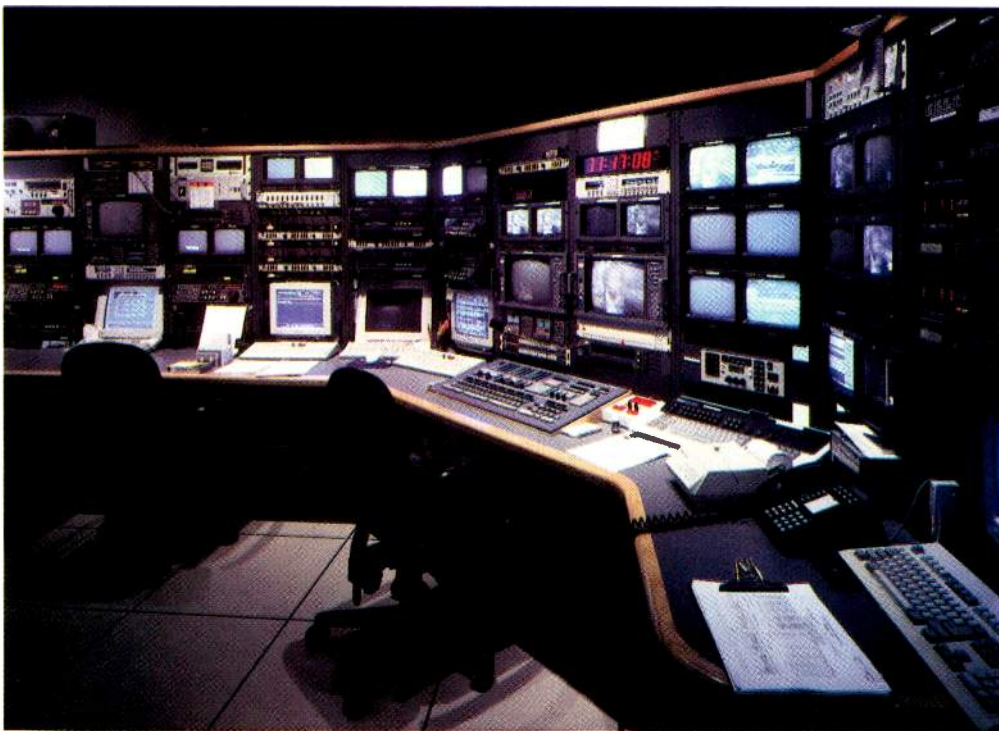
The master control room.
