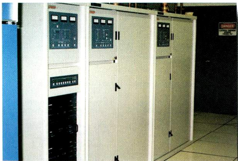
A Harris-Sigma CD transmitter installed at KHOU. (Photo courtesy of Jay Watkins.)
