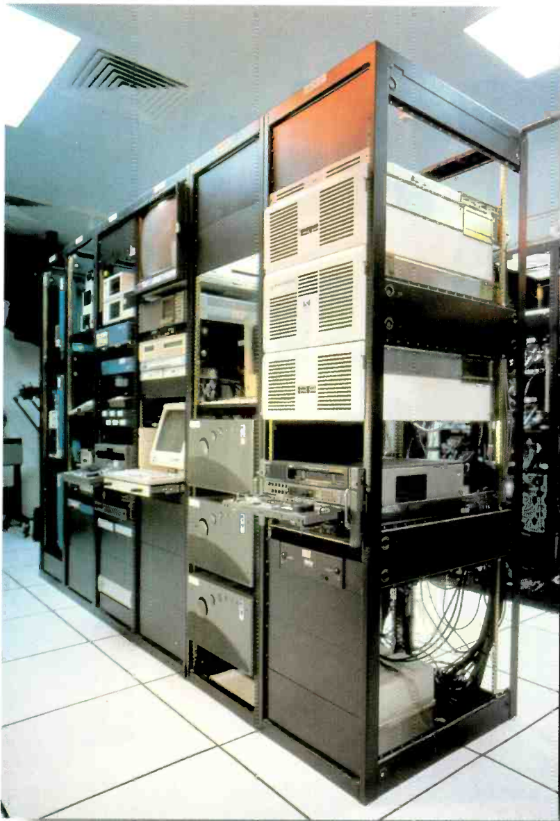
The equipment room showing the Quantel Henry V6, Sony Digital Beta and three Pluto Space recorders.
