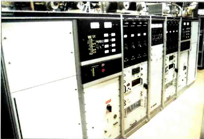
CTN's new Acrodyne transmitter, the Au120D dual-tube 60kW Diacrode transmitter with 120kW output.
