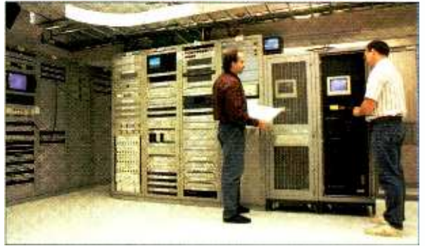
Cartoon Network Brazil is exploring the limits of computers and networking technology. This operation employs traditional 10BaseT networks and FDDI fiber, moving video packets according to commands sent over the slower network. Photo by Mark Hill, TBS, Inc.
