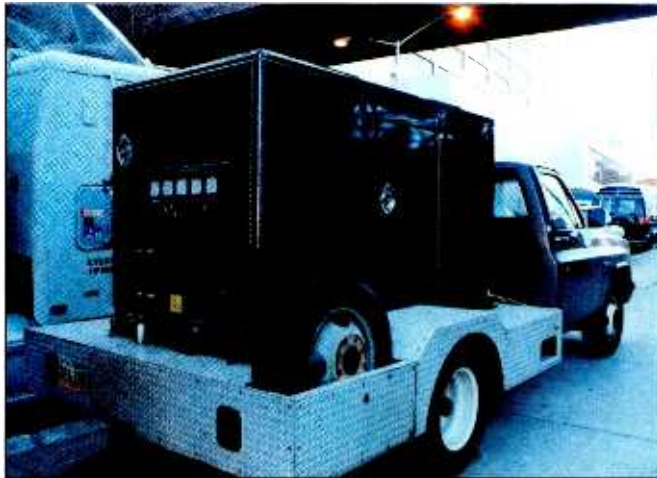
The capacity of this portable, diesel-powered generator is 166A, three-phase (500A total, single-phase). Its housing is felt-lined for quiet operation.
