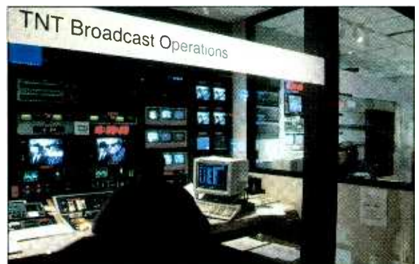
Broadcast facilities like this one at TNT in Atlanta have rapidly assimilated computer and networking technology. Photo by Mark Hill, TBS Inc.
