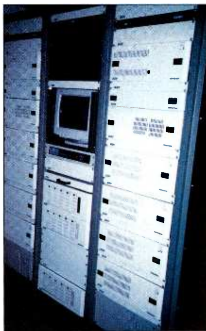
In three racks, this automation system handles spot insertion for 32 TV channels.
