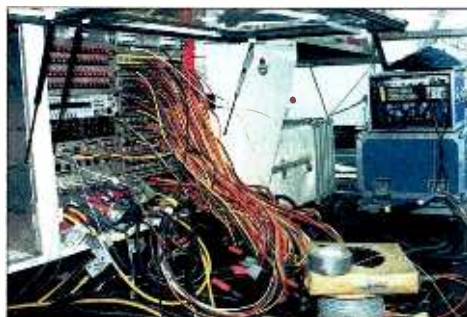
Despite the complexity of hooking up remote trucks, linking their switchers was really quite simple and only required a single cable.
