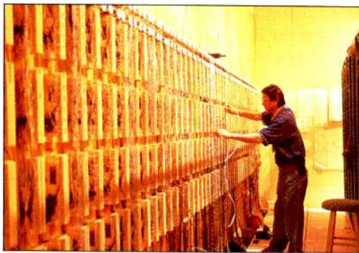
A wall of punchblocks consists of 188 units, allowing the matrix input, output and controlling data cross connecting between the Telex RTS 400x400 ADAM digital matrix intercom system and all the outside venues.
