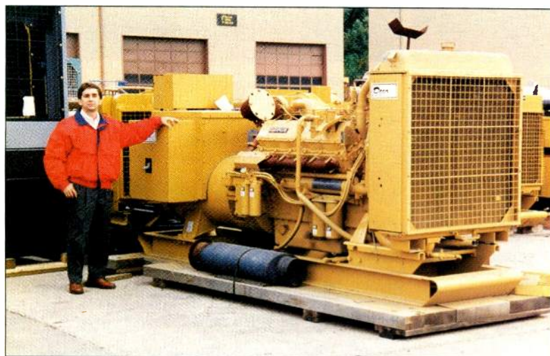
Generators large enough to operate a transmitter facility have significant space, cooling and fuel requirements. According to Mike Batten (pictured), this 12-cylinder Caterpillar can produce 600kW.
