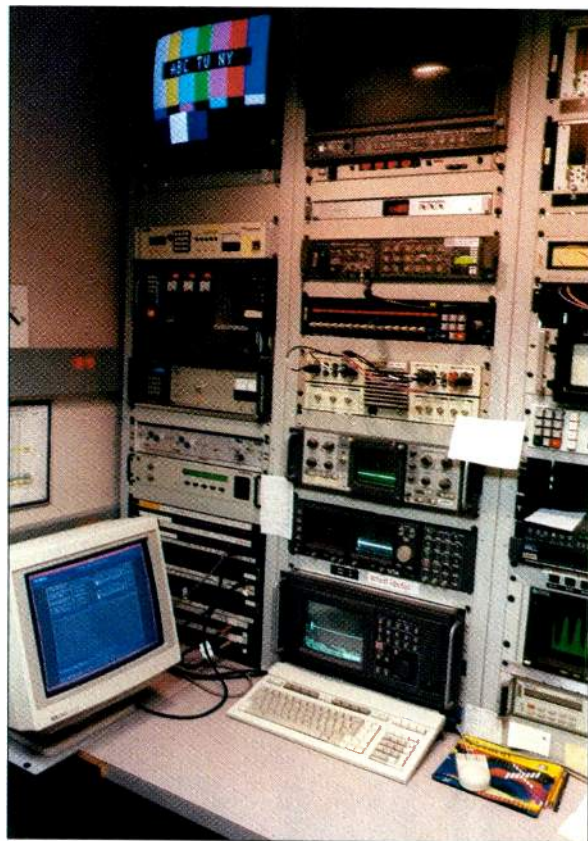
Fully testing all the parameters of audio and video signals requires numerous test setups and a variety of equipment. Shown here is a portion of the test setup in the ABC QC Station in New York.
