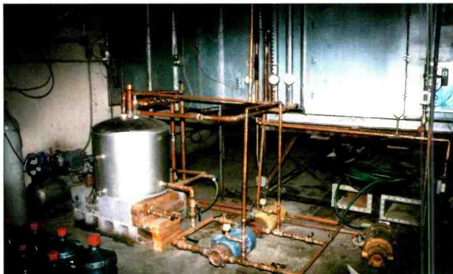
A portion of the heat exchanger along with the pumps and tank used for a water/vapor cooling system for klystrons. (Photos courtesy of David Birdsong, KSMO-TV.)
