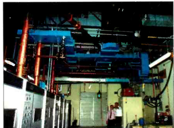
A combiner network using waveguide is common in UHF transmitter installations.
