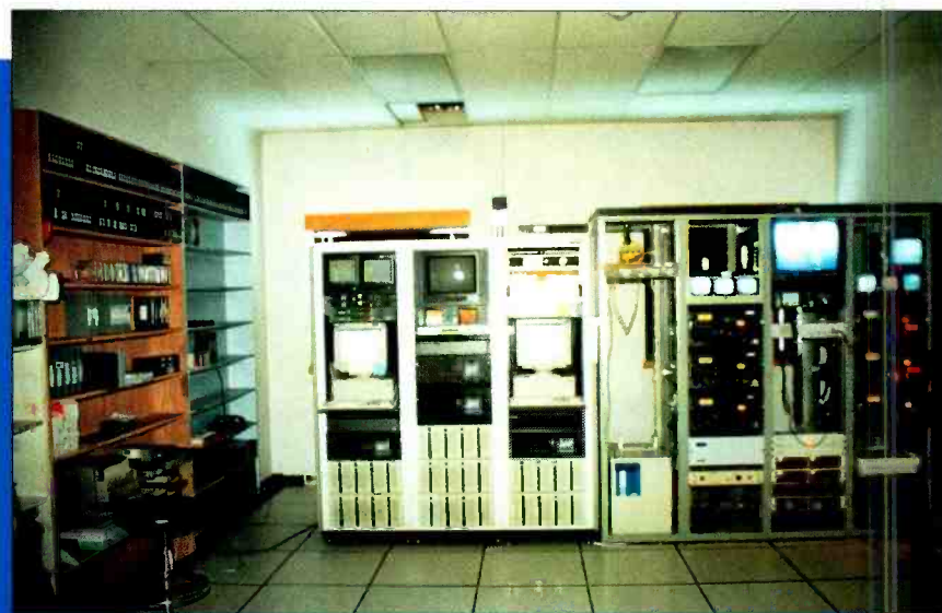
Shown in the mid-construction phase, the Spotbank system at KIMO-TV, Anchorage, AK, is tied to Beta decks for long-form playback.
