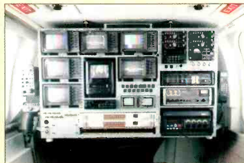
The installation of a sophisticated production system in a helicopter like that shown above, should be handled by experts. Don't assume you'll even know about, let alone, get all the needed FAA clearances.
