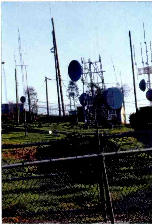
This multitransmitter microwave site has no warning signs posted.
