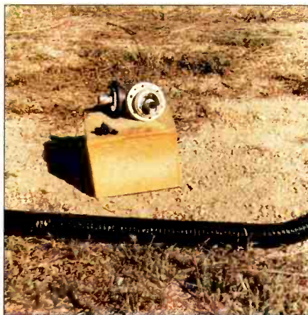
This broadcast line was struck by lightning. The coax was destroyed — even the outside plastic jacket of the coax was melted. The black, charred piece next to the elbow is a melted bullet.
