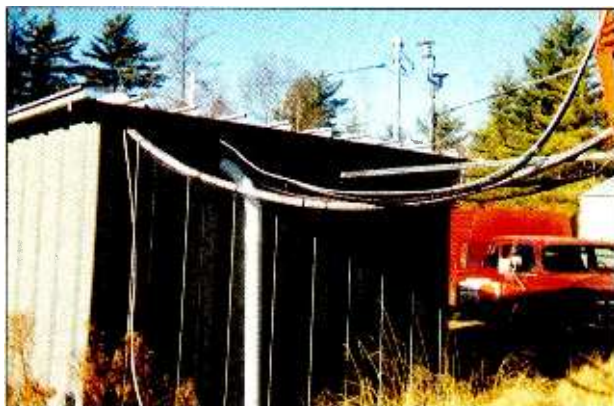
An example of how not to do things. One small ice bridge is used to protect one transmission line. The remaining lines are unsupported and unprotected between the tower and building.
