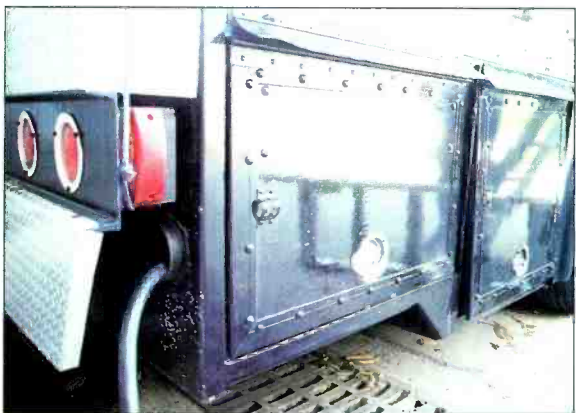
At top, this production truck's power bay has been hastily hooked up to mains incorrectly. Center photo shows the proper hook up, routing cables through duct on left side of power bay. This allows the power bay door to be completely shut (bottom photo), providing increased safety and security.
