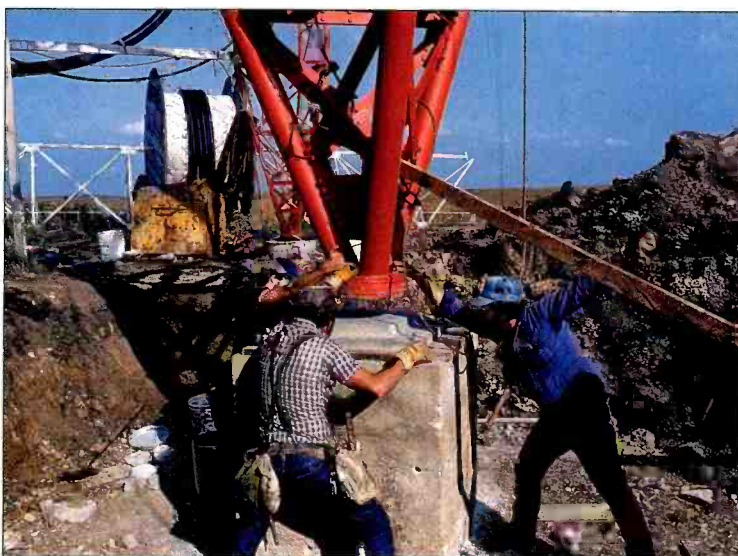
KLDH-TV transmitter site September 1984. Setting bottom 150-foot section of replacement 1,439-foot tower. Note standby 400-foot tower in background. Tower crew is placing bottom triangle section on main pin on base plate.
