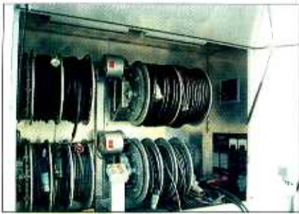
Power take-up reels in the back of the 46-foot trailer. Motors simplify the job of winding and unwinding cables. (Photos courtesy of Georgia Public TV.)
