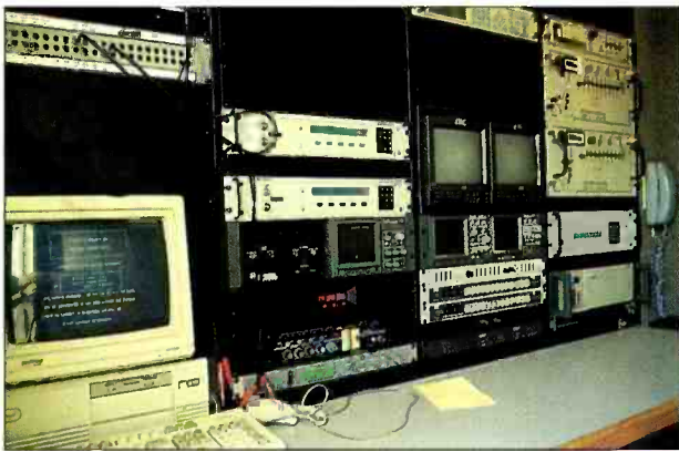
Interior of the uplink trailer shows plenty of room for expansion if needed.
