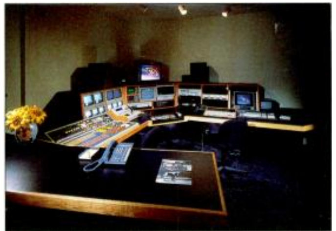
Careful layout of operator-intensive controls, as shown here, makes this on-line suite convenient and ergonomically friendly.
