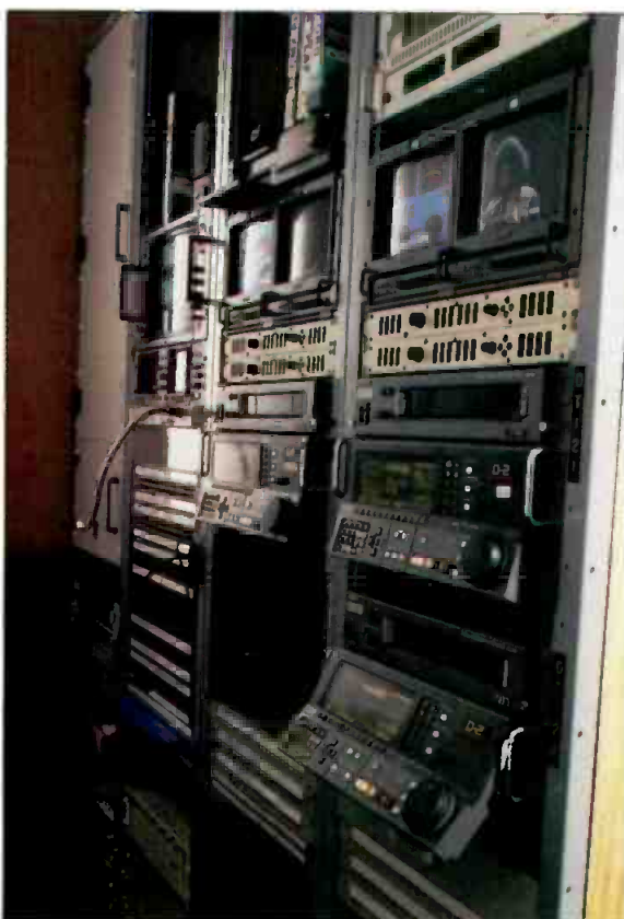
Racks in the equipment room that contain tape machines and electronics used for Edit 12.
