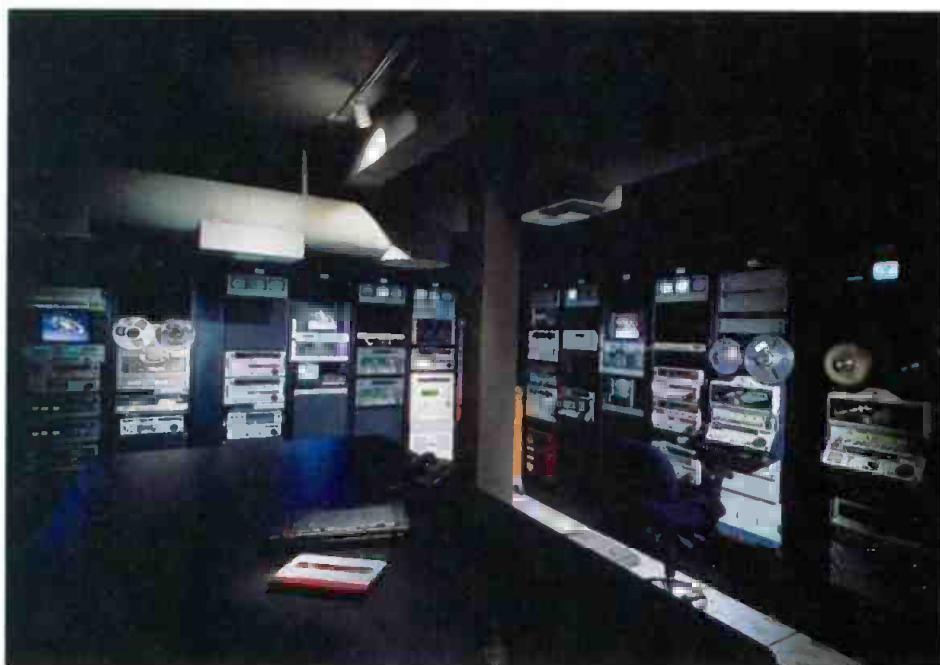
The master control room incorporates several unique features, including a highly efficient HVAC system and direct signal routing to all edit suites.
