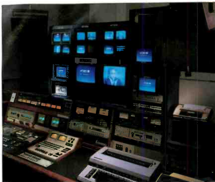
KQED's new on-air control room was the first new area to begin operation during the phased relocation.
