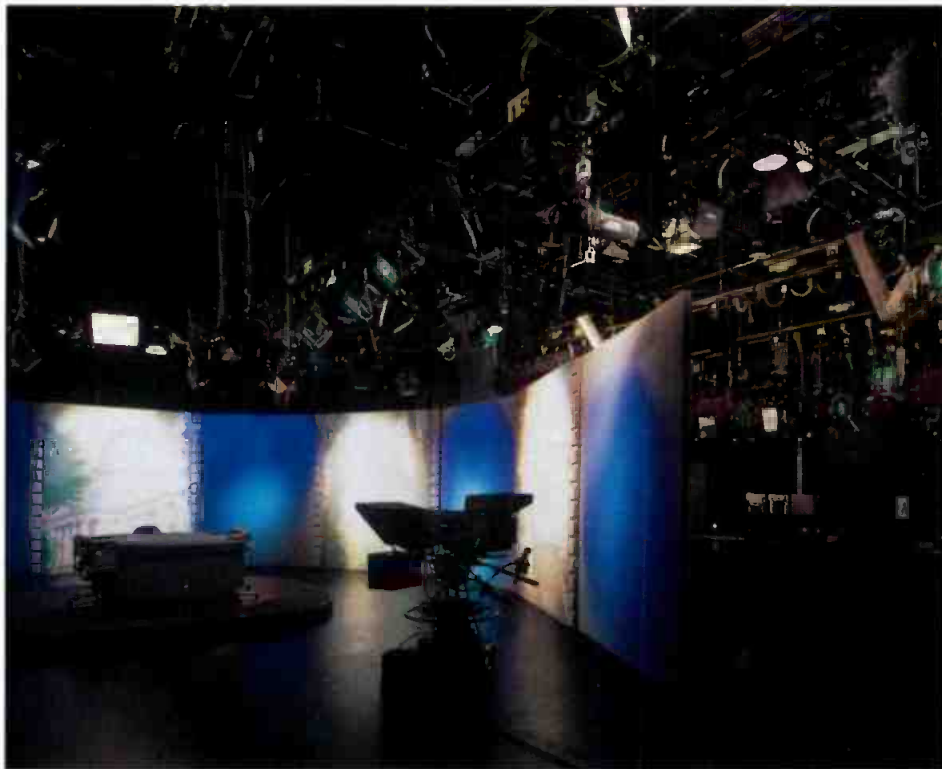
KQED's Studio A, a 4,000-square-foot studio for large productions, features a unique bilevel air distribution system and a fully motorized lighting batten system.
