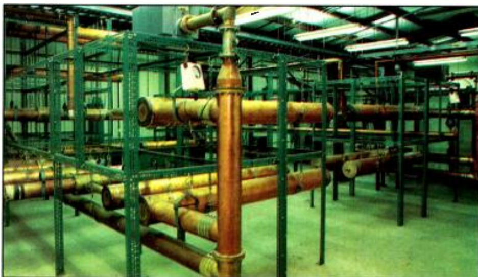
The multiple FM transmitter combiner network at WBNS, Columbus, OH, handles signals for five high-power stations.
