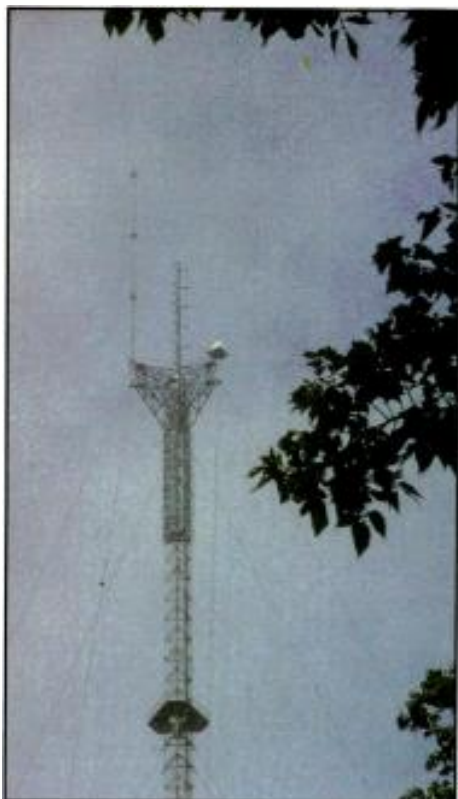
A candelabra on the top of the WBNS tower (Columbus, OH) holds the WBNS-TV and WCMH-TV antennas and an ENG receive site. A multistation FM panel antenna is mounted just below the candelabra.
