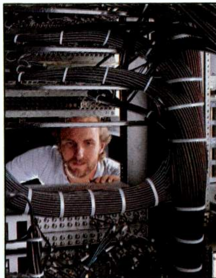
Neatly bundled and marked cables aid in troubleshooting and create a favorable impression on prospective clients.
