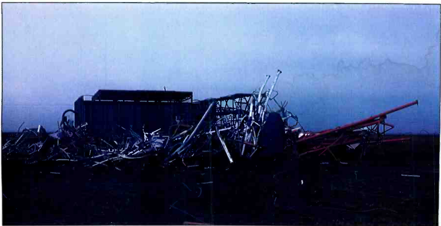
The failure of this tower was caused by either poor design, poor maintenance, or both. This problem could have been avoided.
