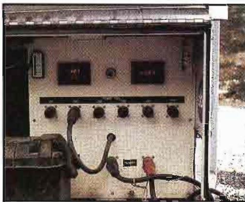
A typical RPV power panel. Note the digital readout of voltage and line frequency.
