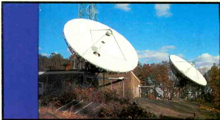
Two terminals at the PBS MOT at Bren Mar, VA, link to Westar IV for program distribution to the network stations.
