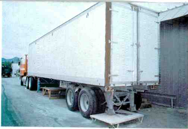
Rear view of van approximately two weeks into construction. Note special level landing gears in place.
