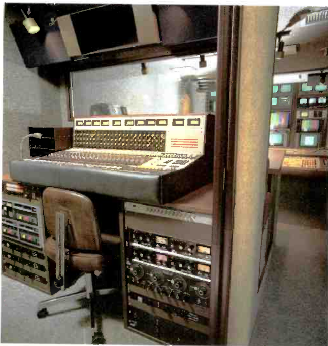
The audio booth (foreground) is a stand-alone unit but interconnects to the production area (background).
