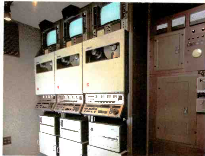
The videotape area faces the video terminal space. It contains a breaker box and custom-designed tilt-out transport mounts. Each machine has full monitoring capability.
