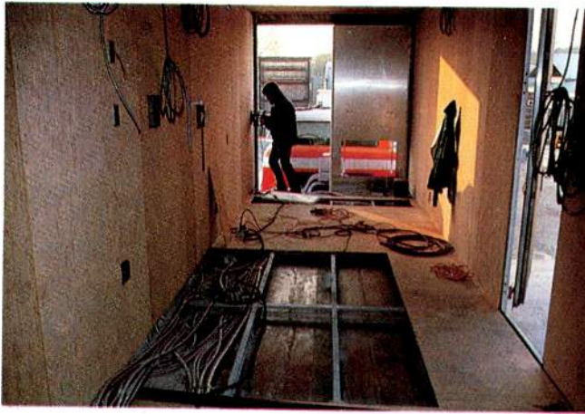
Raised subfloor provides space for wiring of systems.
