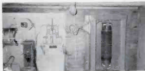
Fig. 3 This antenna tuning unit was completely under water.
