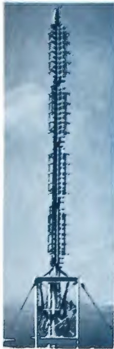
Directional VHF-TV Transmitting Antenna
