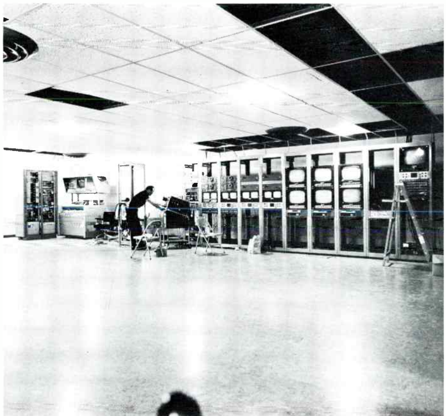
Fig. 2. Spacious master control room serves origination studios of network.
